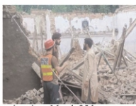
rains since March 25 have caused roofs and walls of houses to collapse, resulting in 17 deaths and 56 injuries. Among the deceased were 14 children, one man, and two women. According to the report, 11 houses were damaged due to the rains, with most of the incidents occurring in Bannu and North Waziristan. Meanwhile, the Pakistan Meteorological Department.
